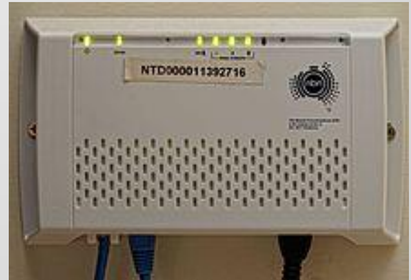
Network Termination Unit
