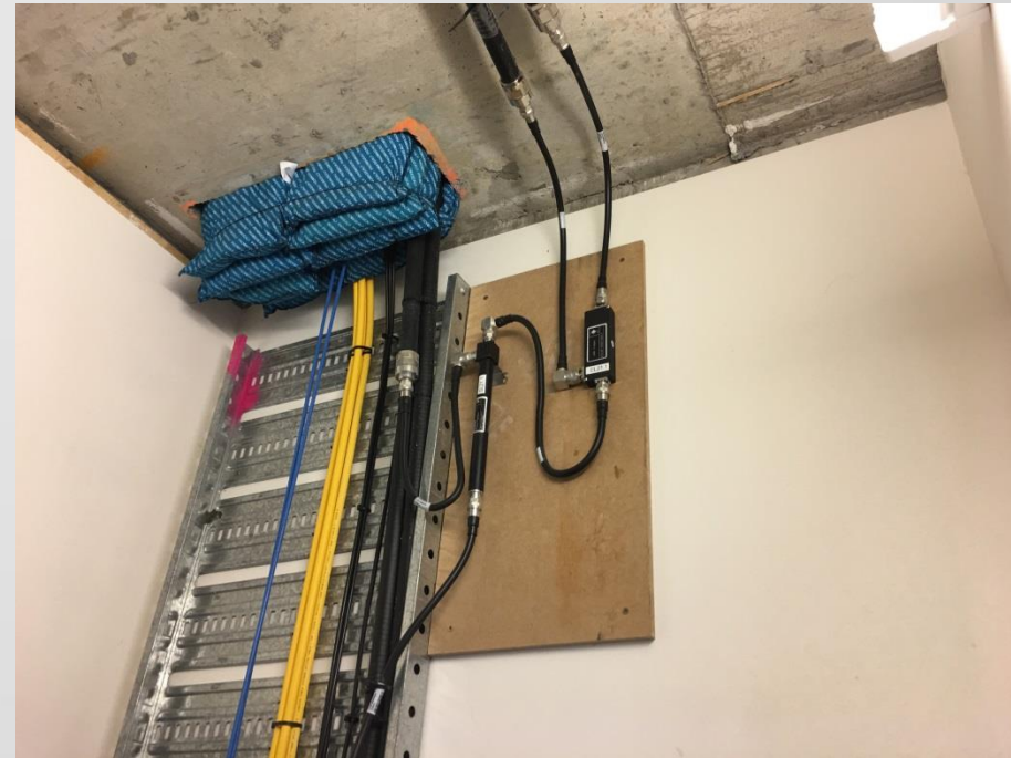
Fibre Run Between Floors
