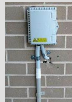
NBN Utility Box
